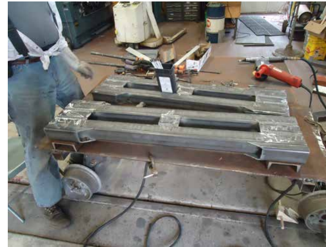
Completing the welding of the spring planks for the RPO trucks in the CRF
