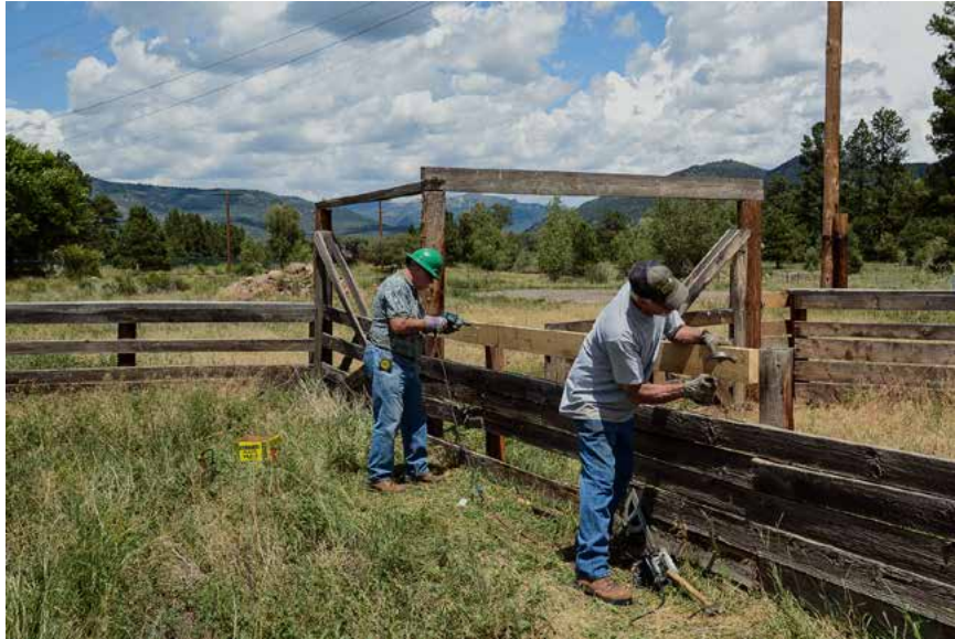
At the other end of the yard Len Jones and Jim Herriott are making repairs to the stock pens.
