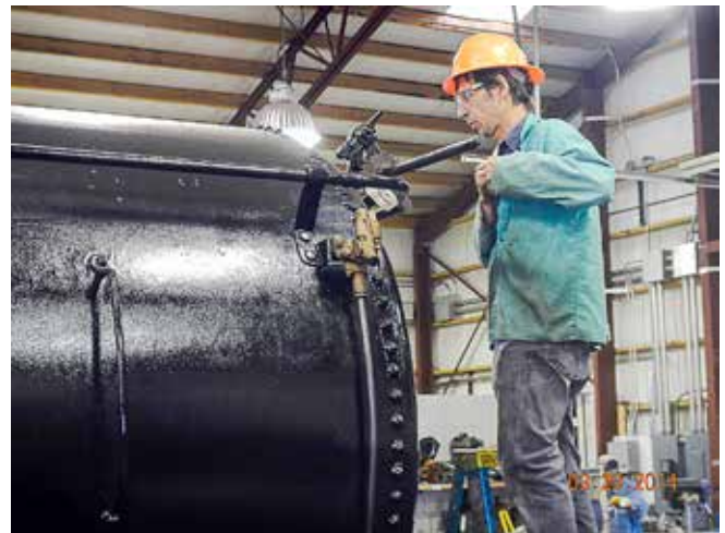
Chris Trunk is replacing missing tank car jewelry - this is prep for the brake wheel.
