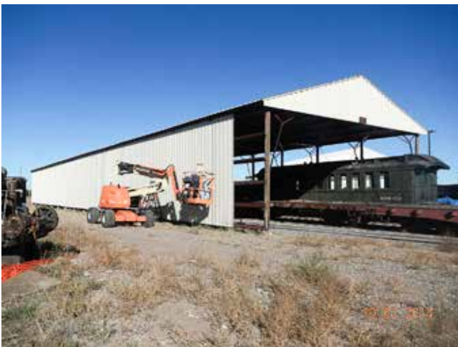
Car shelter siding completed - well missing two pieces.
