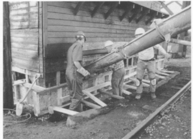
Team Leader John Sutkus, Don Bayer and Bob Conry pour concrete into the forms.
