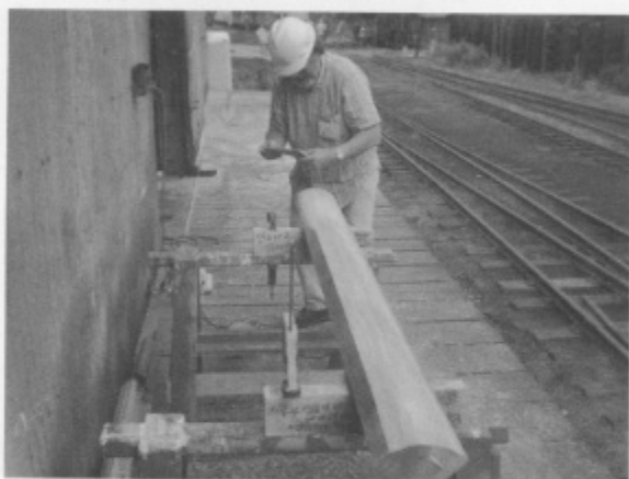
Bill Jacobs uses a template to check proper curvature of a corner post. There are a total of 12 corner posts, six on each side. Nine new posts had to be made as only three were salvagable.
