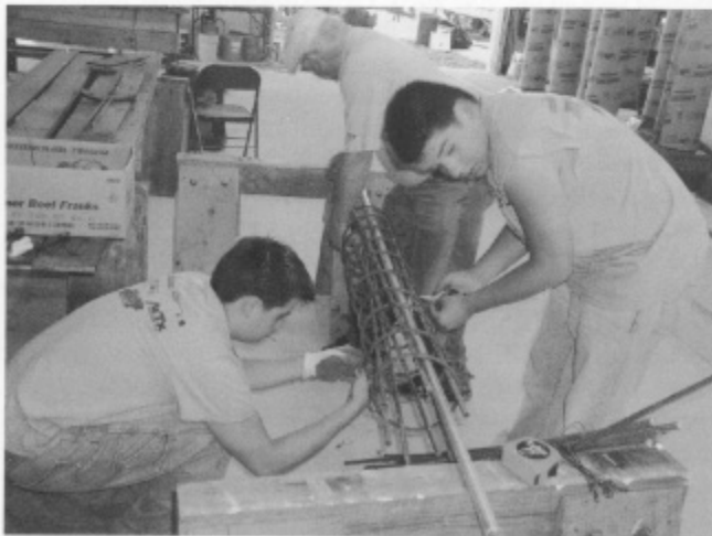
Daniel and Guy McGonagle wire tying cylindrical rebar cages for pole footing reinforcement.
