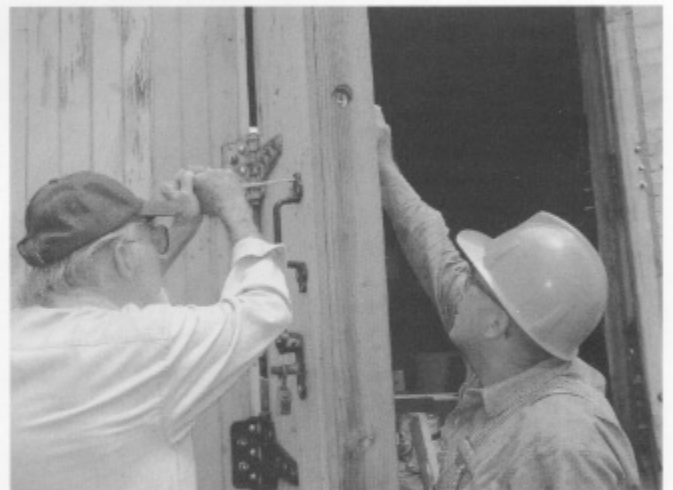
Richard Howell and Matt Jameson installing hardware on a door of the reefer.
