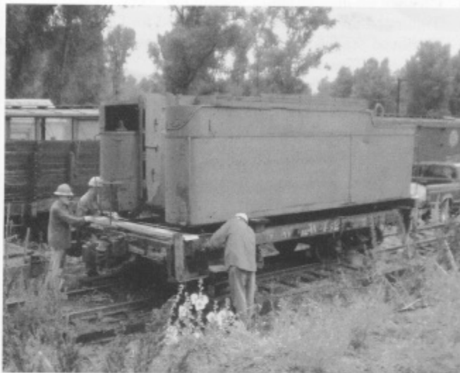
Water tank has been jacked up in preparation to install the new floor.
