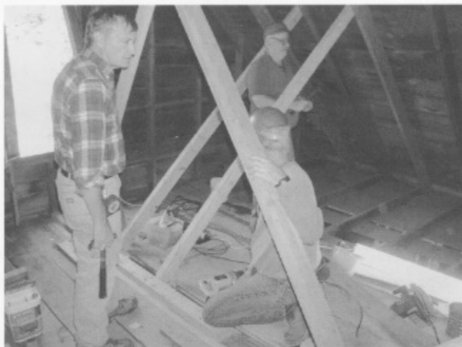
Dave Ferro, Andy Hackmeyer, and Tom Gregory bracing the roof of the Car Inspector's house.
