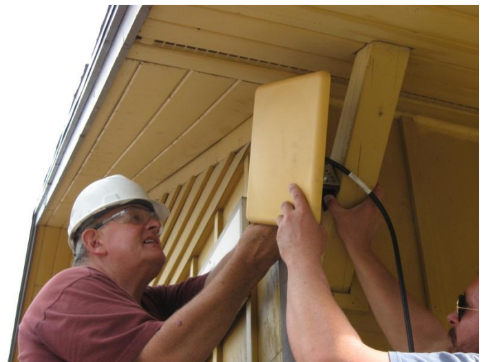
John Eng and Joe Kanocz mount an antenna to the bathroom building
