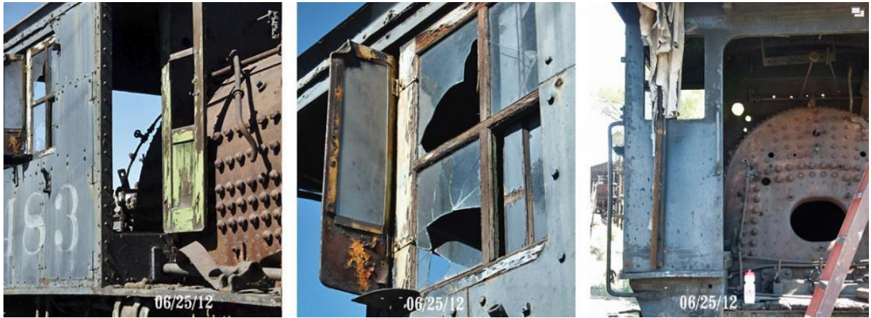
Various pictures of 483 deterioration through the years taken by Russ Sperry.
