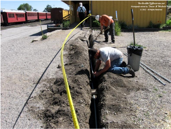
John Eng and Joe Kanocz lay PVC in the newly dug trench between the Depot and bathroom building
