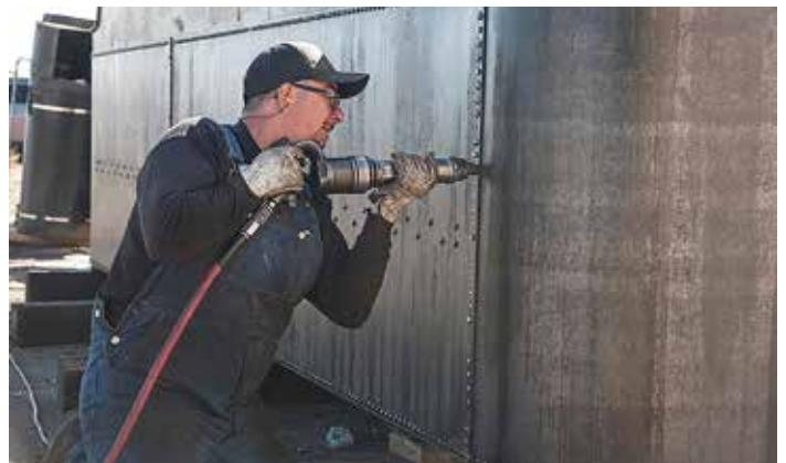
Weather had damaged the tender and the cab beyond repair so a replica tender was built in Antonito. Stathi Pappas secures one of the new tender's 1,600 rivets.
