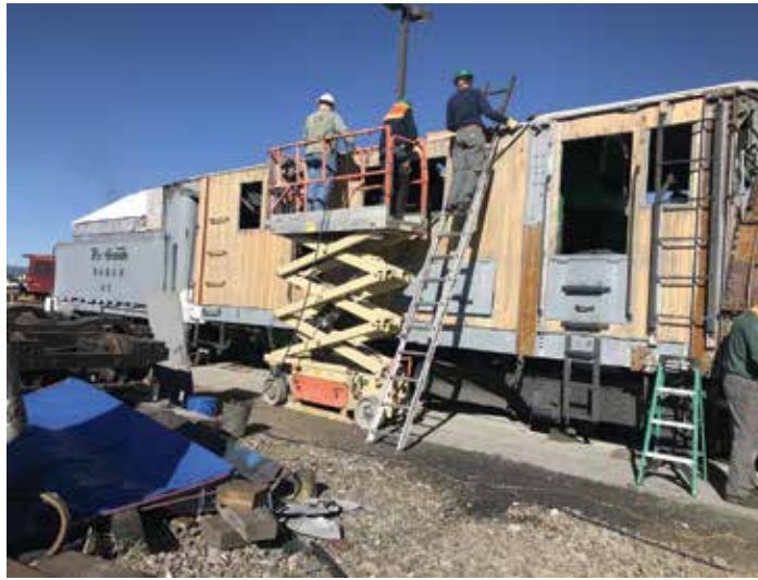
Bryce Templeton, Don Atkinson, and Keith Anderson work on the roof from the scissor lift.
