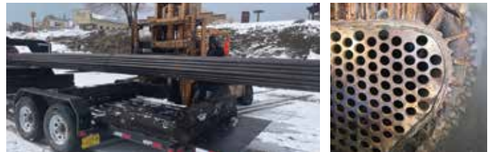
The 152 new boiler tubes arrive from Germany to be installed in the flue sheets when repairs are complete.
