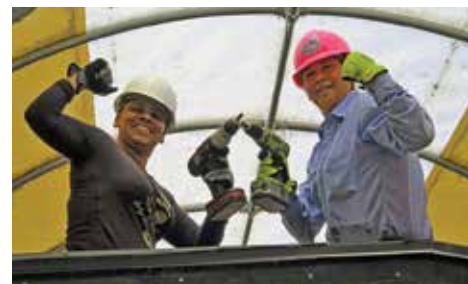
"We can do it!" Like modern day "Rosie the Riveters," Mavy Chararria and Norma Lock work on the roof of a sheep car in the work tent below the Chama Roundhouse.
