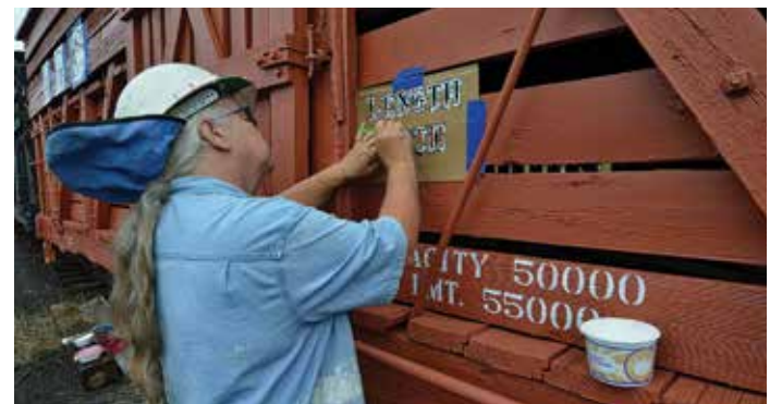
Restoration doesn't stop with reconstruction. The stock cars also have to be repainted and lettered accurately. Patty Lounsberry adds reporting marks on a restored stock car, lettered for the Rio Grande Southern. Photo by Friends Chronicling Team
