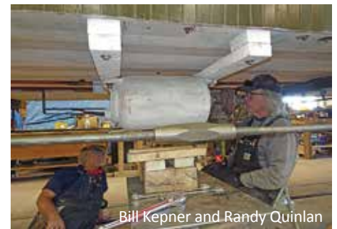
Bill Kepner and Randy Quinlan inspect the air reservoir near the center of the Car.
