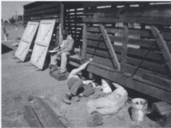
Team Leader Dan Pyzel taking notes as Mike Horner and another team member work underneath the car.
