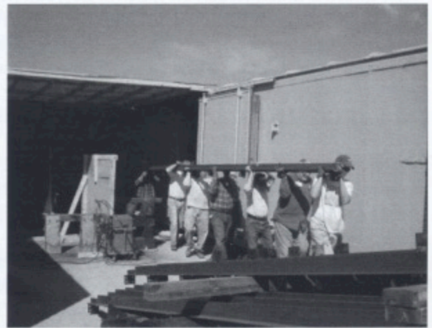
Team Leader Russ Hanscom, Tim Bristow, [unknown], Bob Reib, Bob McCain, Marshall Smith, and [unknown] carry a welded truss chord to be stacked on the trailer.
