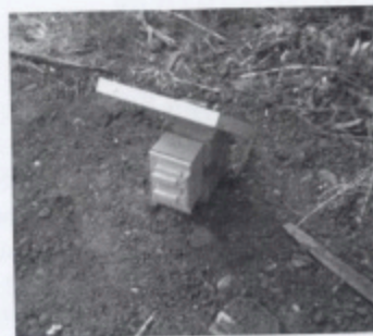
Close-up of one of the two temporary electrical outlets.
