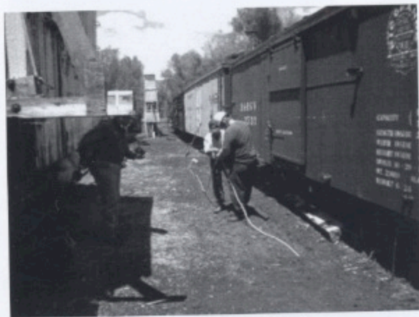
Bob McCain and TL John Engs splice the temporary electrical line to the north outlet.
