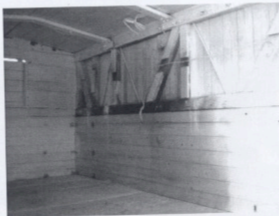
New electrical Romex wiring hanging from the ceiling and along the wall.
