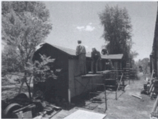
Larry McDonald, Team Leader Phil McDonald and Fred Morton putting down new green mineral roll roofing.
