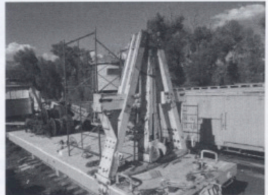
The double drum winch assembly has been moved back onto the car and the pivot post has been secured.
