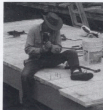
Team Leader Russ Hanscom using a short handled "8 pounder" to nail the 40d ring shank nails into prior drilled pilot holes.
