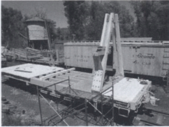
Decking has been notched underneath where necessary in order for it to lay flat when nailed in place.
