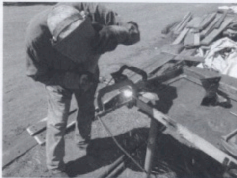
Marshall welding retractable wheels on the band saw base for easier movement inside the carpentry shop.
