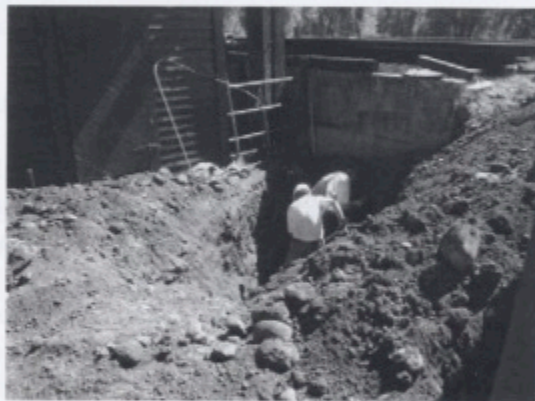
Against the hoist house is the lightning protection ground loop.
