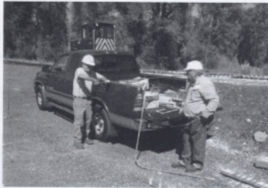
Gene and Bill Bailey working on the ground loops for the north and south side of the hoist house.
