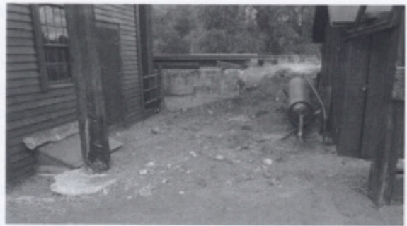
Lightning protection ground loop and ground enhancing material has been installed and the hole backfilled.
