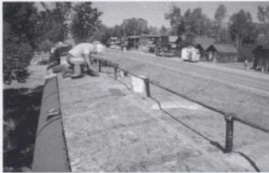
Chuck Deuker puts temporary repairs on the roof of Car No. A-3.
